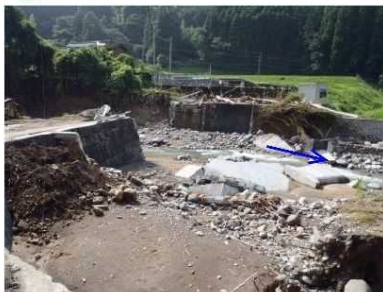
② 橋梁被災(流失)状況(小園橋)
